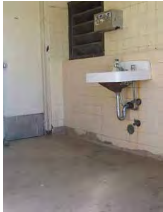
Image 39: Park restroom in need of renovation.
